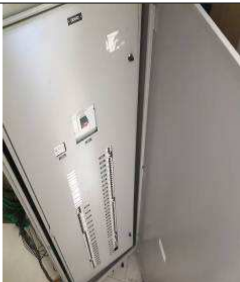
Figura 37E: Quadro QD-AR3 (lateral VM362)
