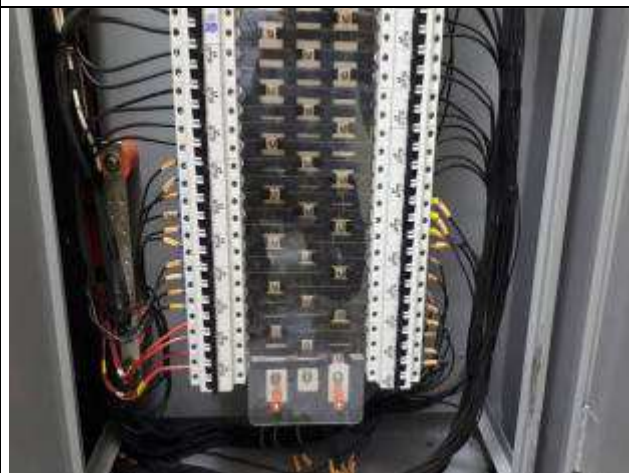
Figura 40E: Quadro QD-AR3 (lateral VM362)
