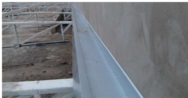
Figura 15C: calha instalada no bloco central (frontal)
