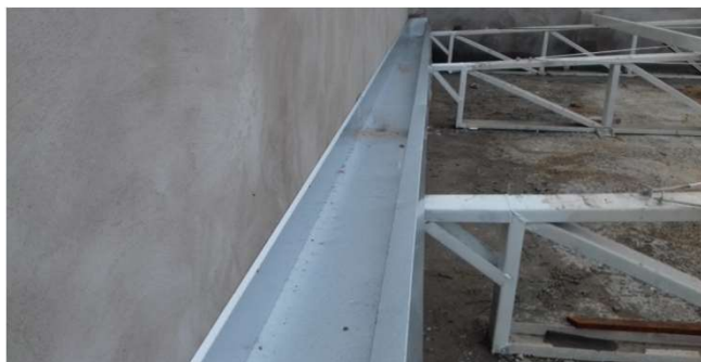
Figura 14C: calha instalada no bloco central (frontal)
