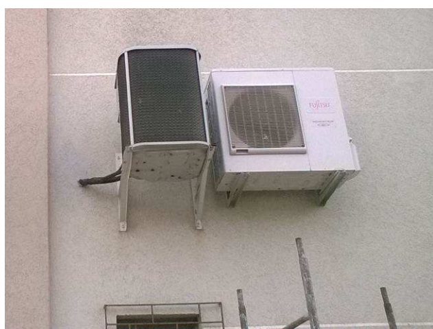
Figura 22C: Condensadora 1 - Service Desk.
