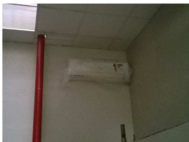
Figura 21C: Evaporadora 1 - Service Desk.
