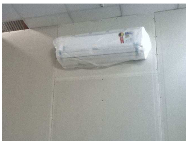
Figura 23C: Evaporadora 2 - Service Desk.
