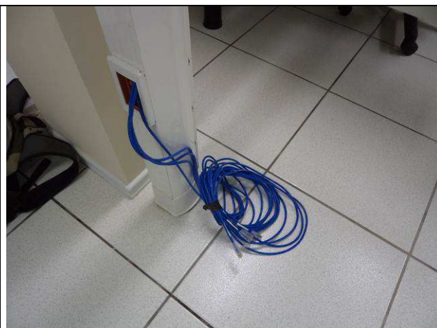
Figura 58E: patch cords de 10,0m.
