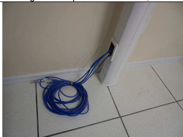
Figura 59E: patch cords de 10,0m.
